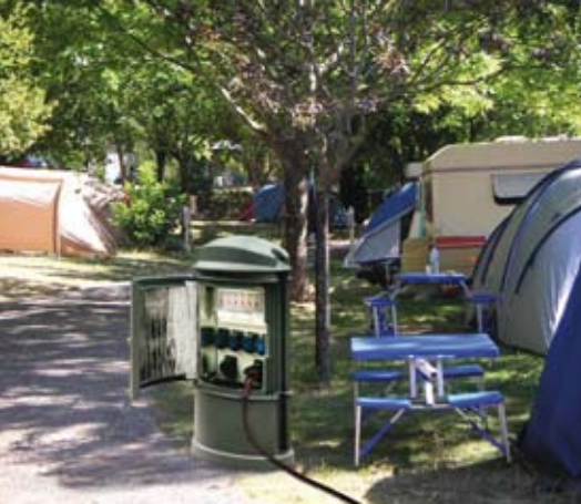
fixed power dispensers
